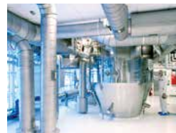
PHARMA-SD® type PSD-4 drying chamber and HVAC ducts.
